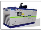
DG Set For Power Back Up
